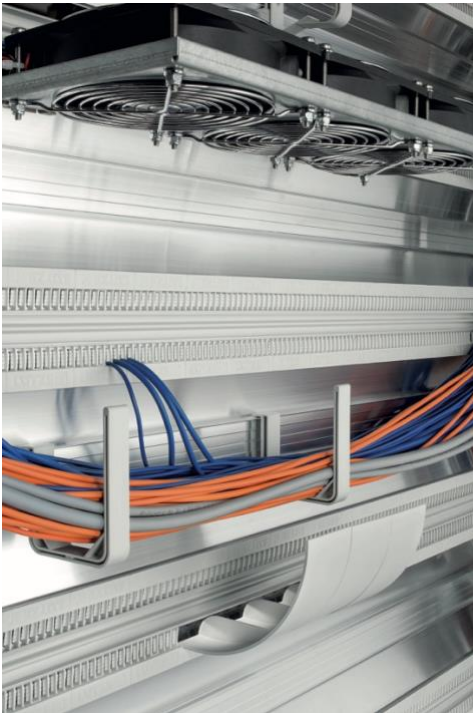
Figure 4: Airstream wiring with the Airblower fan (Lütze)
